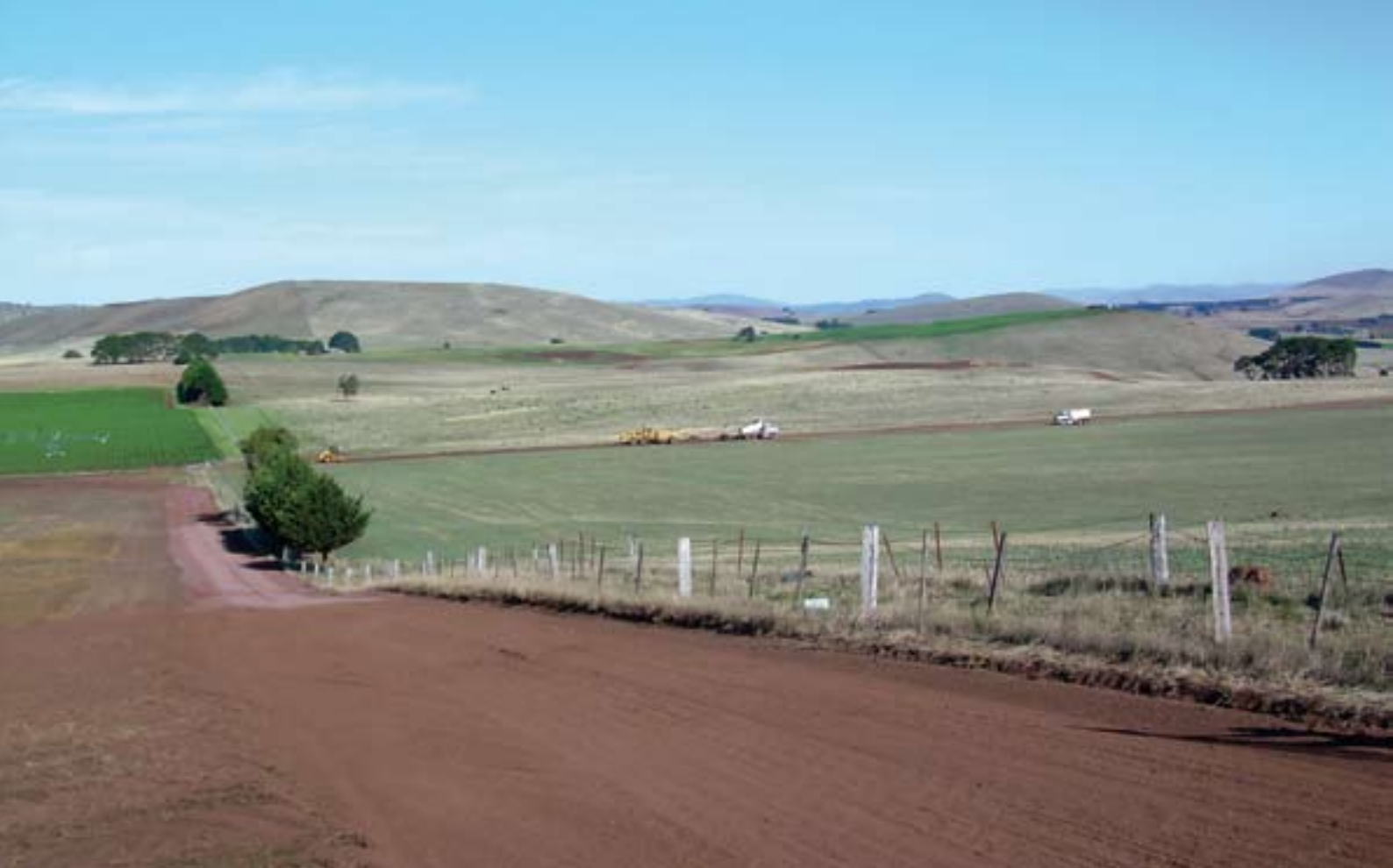
Construction in progress A turbine access track being built (above), the main pour to a turbine footing (below left) and checking the steel frames for a turbine foundation.
